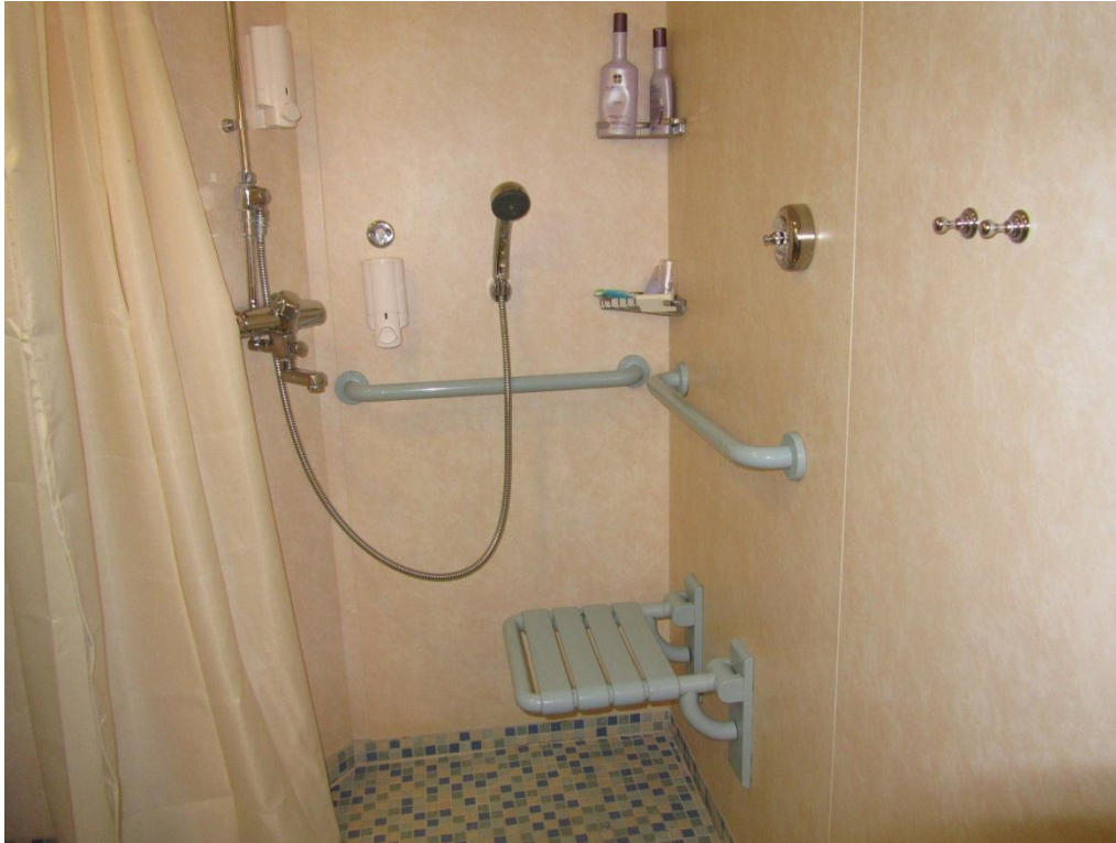
Figure 2 Accessible Roll-In Shower
