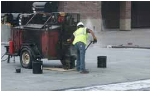
Hot rubberized asphalt melter
